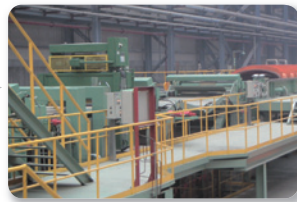
酸洗线 Push-Pull Pickling Line
