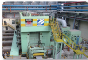
酸连轧线/PLTCM Pickling & Tandem Cold Mill
